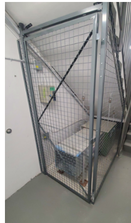
Press Fan and Stairwell Fencing with Access Door
