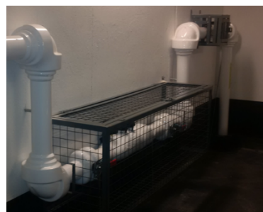
Pipe Enclosures with Access Doors
